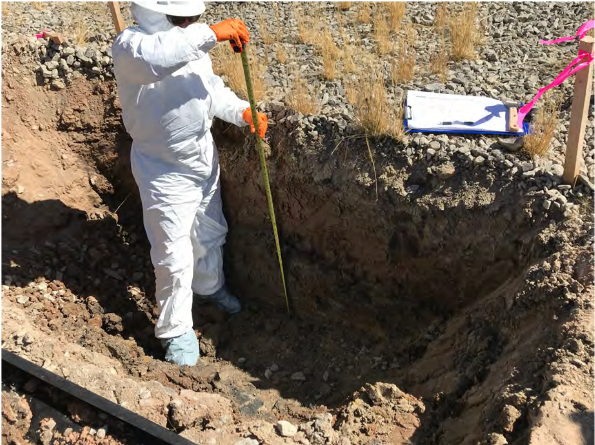
Photo 27. Emily Woolsey (INTERA) measuring depth of UT-TP1 test pit at 3.6 ft. Cover profile contains moist clay and shallow grass root systems with highest root density within the top 8 in. Tyvek suits were worn in the first two tailing test pit excavations then reduced to only Tyvek booties as no elevated material was encountered within the cover materials.
