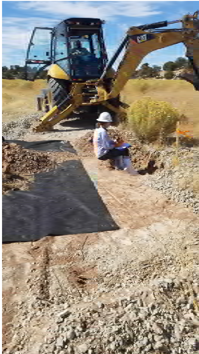
Photo 21. LT-TP1 test pit excavation. At all four test pits on the tailing impoundment cover, the limestone cover rock within the work area was scrapped into a stockpile and cover material was placed on soil cloth in separate piles in order of excavation depth to recreate the cover profile after investigation. Tailing test pits were excavated in stages to document the shallow cover soil profile before digging deeper into cover material for ALARA exposure purposes.
