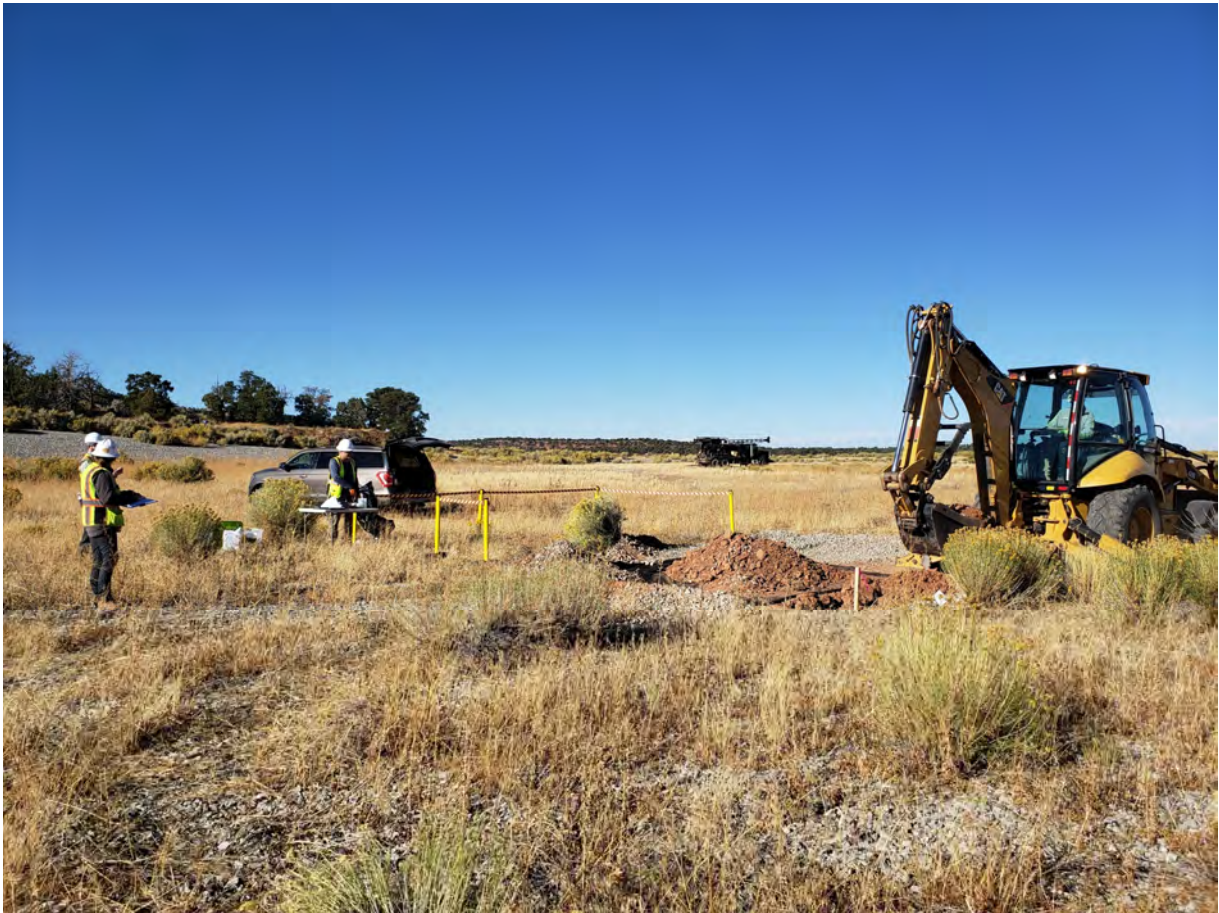
Photo 24. Excavation scene at LT-TP2 test pit showing work area exclusion zone set up by ERG and typical distance maintained from test pit during active excavation. Vegetation at LT-TP2 includes rubber rabbitbrush, yellow sweetclover, redstem filaree, and grasses (Foxtail barley, wild oats, and cheatgrass).
