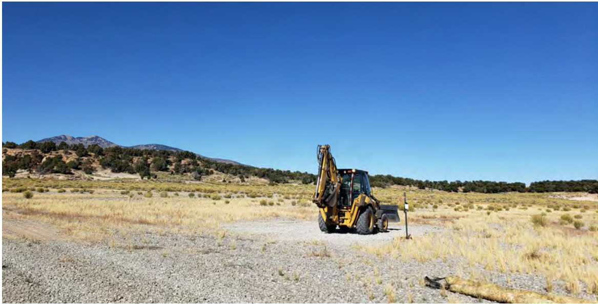
Photo 28. Forrest Waggoner (DalMolin) spreading and compacting limestone cover gravel over backfilled UT-TP1 test pit.
