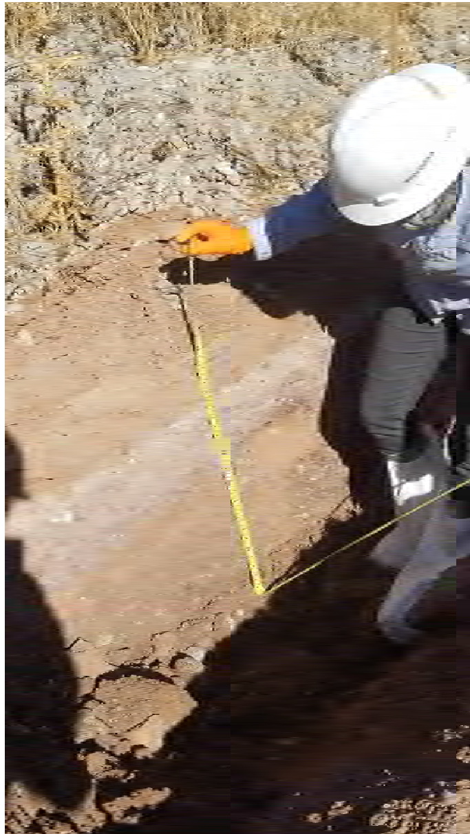
Photo 23. Cover soil profile at LT-TP1 test pit showing a greyish-purple silty sand and gravel layer from 1.5 ft to 2 ft depth.
