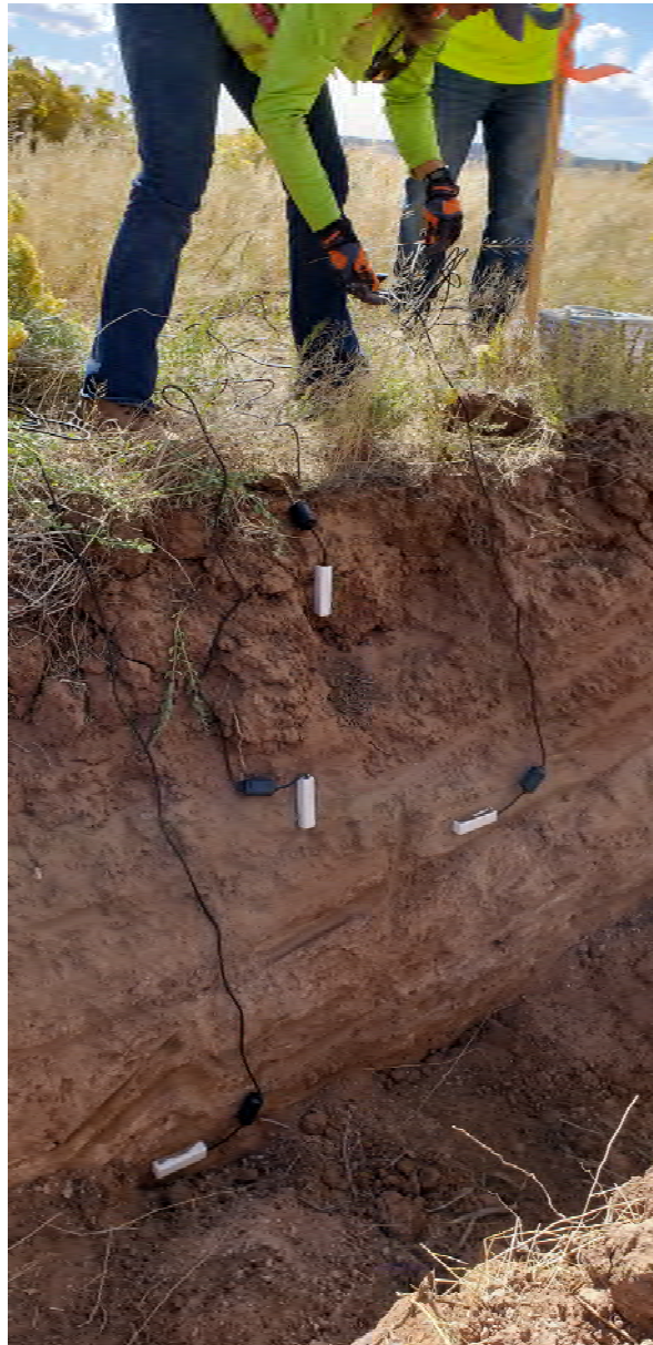
Photo 15. Annelia Tinklenberg (INTERA) installing soil moisture sensors in the NR-5 test pit. The highest root density occurs within the top 1 ft. The bottom of the test pit at 3.5 ft consists of silty sand with pebbles and cobbles up to 1 ft in length.
